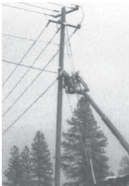
. . . and restoring service
